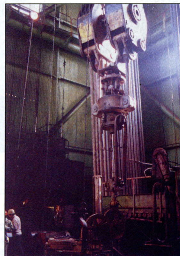
Inside the drilling tower. The lifting gear takes the 180 ton weight of a 12 km long drill string.
